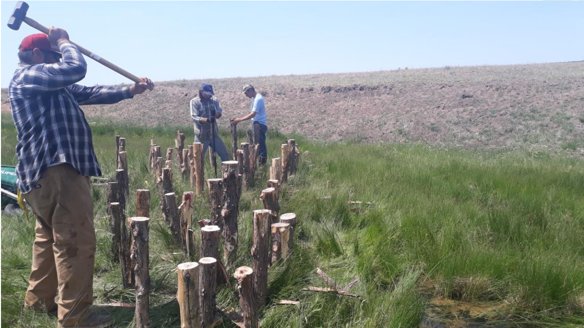
Figure 7. Construction of Juniper wood pole Baffle, built to induce meandering of bankfull flood flows.
