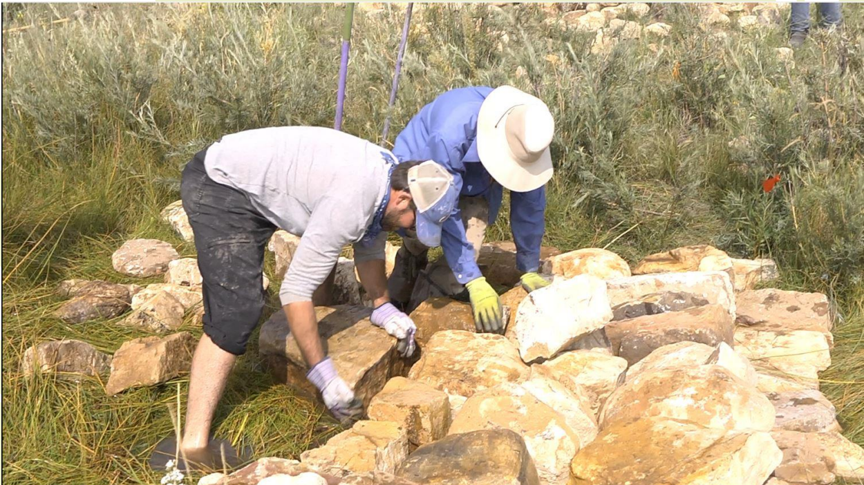
Figure 10. AWF volunteers constructing ORD structures one rock high across the active channel.
