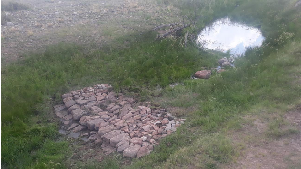
Figure 9. One Rock Dam structure built across the width of the bankfull channel on Wolf Creek.
