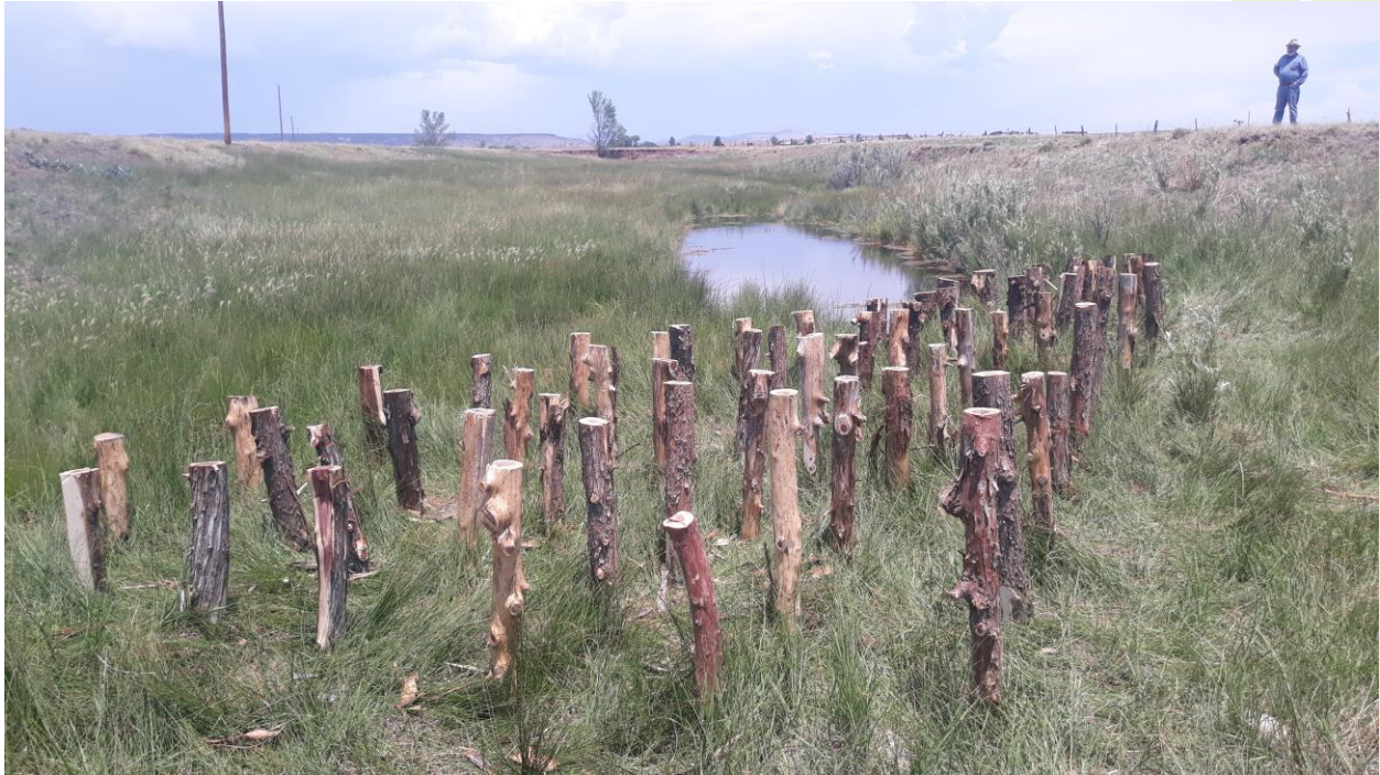
Figure 12. Baffle structure to induce bankfull flows to erode the meandering bank and increase length.
