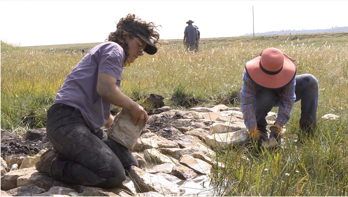
Figure 9. AWF volunteers constructing ORD structures across the bankfull width of the active channel.
