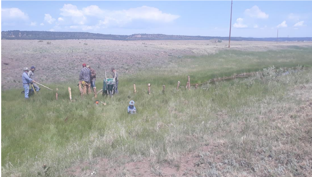
Figure 5. Bill Zeedyk directing the construction of a juniper pole baffle on Wolf Creek.
