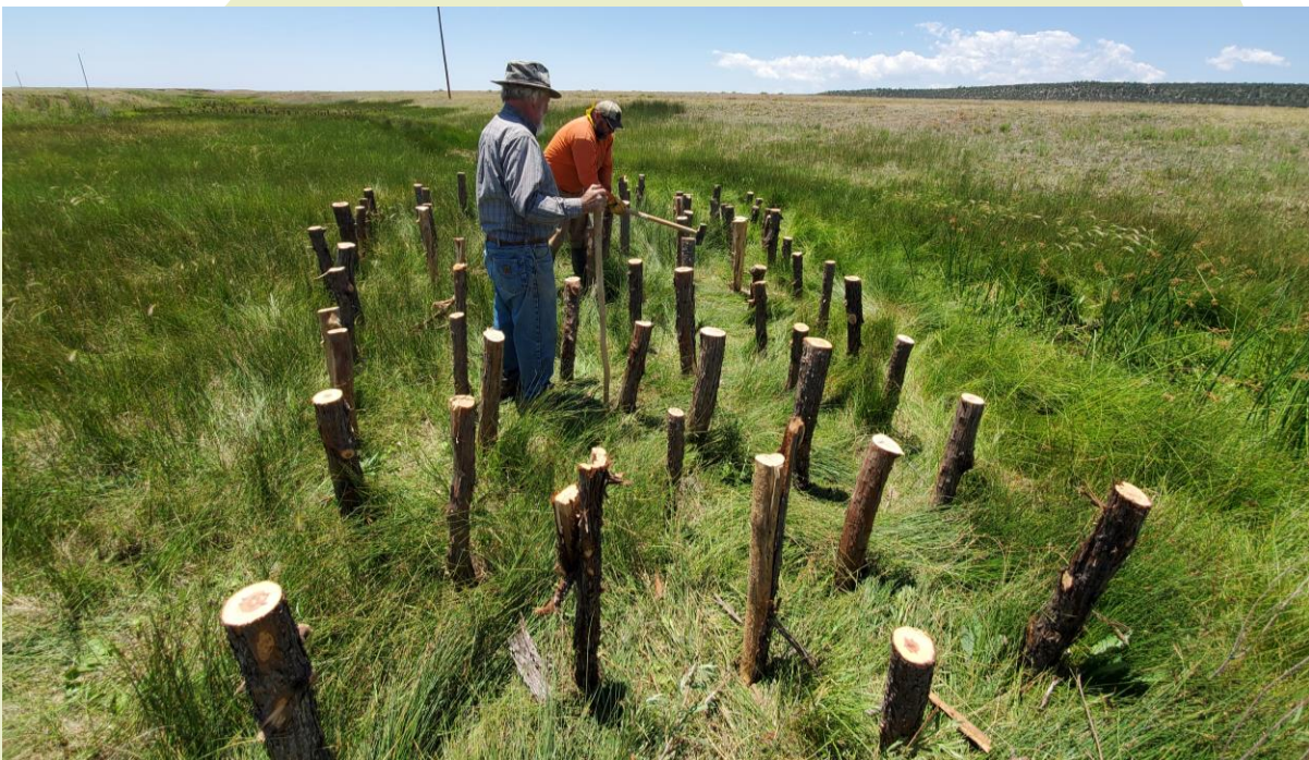
Figure 8. Bill Zeedyk directing the height of the baffle pole as well as the spacing and angle of the structure.
